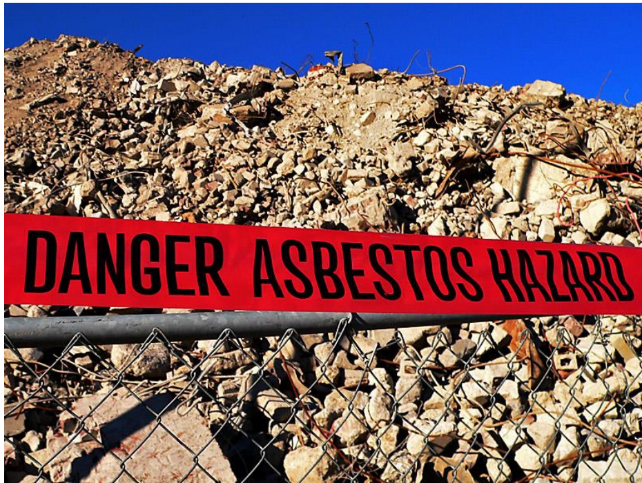
Danger Asbestos Hazard by Matt Niemi | Flickr | CC BY-NC-ND 2.0
